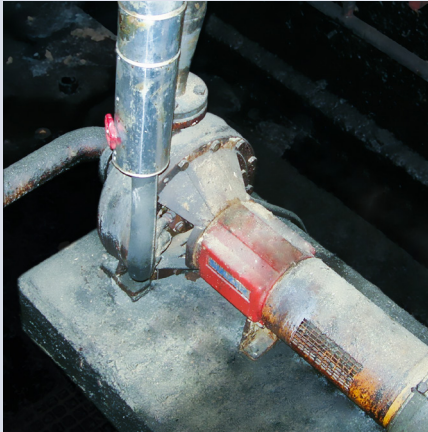
The tall oil pump equipped with a Mtex cartridge seal at UPM Pietarsaari
